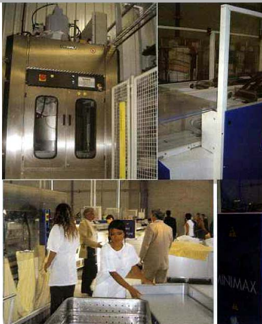
The complete Girbau-Jean Michel equipment has been installed in the Grenat Laundromat
